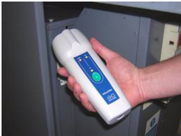
Red Indication Pointing Towards Switchgear
