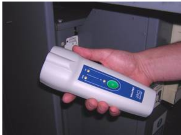
Green Indication Pointing Away From Switchgear
